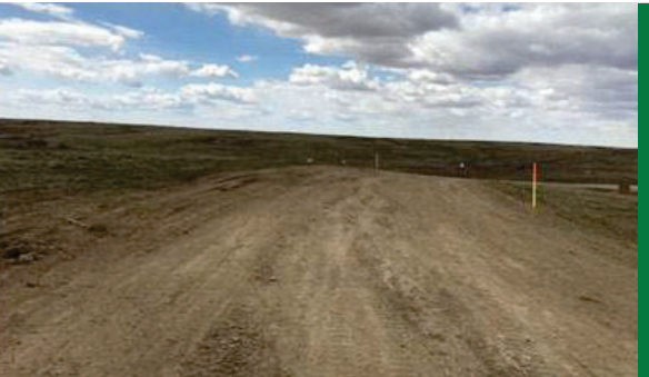
Once the impacted soil was successfully excavated, the impacted area was backfilled and recontoured with a soil with similar physical and chemical properties to those found within the region.
