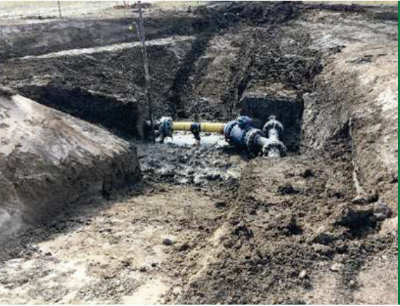
The exposed breakpoint is evident at the base of the pipeline excavation.
