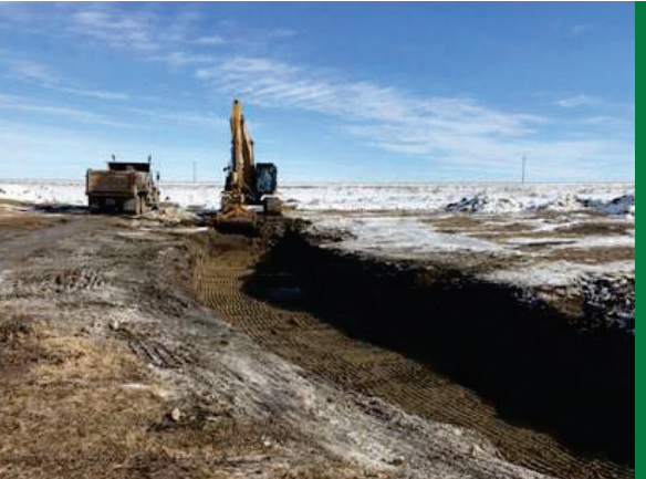
In 2020 the remaining surficial impacts were excavated and disposed of at an approved waste management facility during frozen ground condition to minimize damage to the native pasture.
