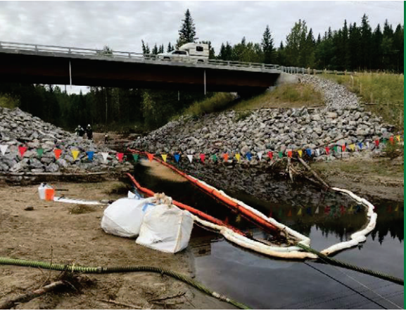
An accessible containment site located down gradient of the point of release.
