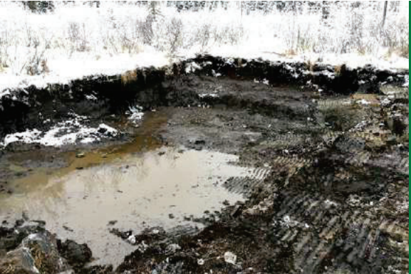
Heavily impacted surface soils were excavated and disposed of at an approved waste management facility.
