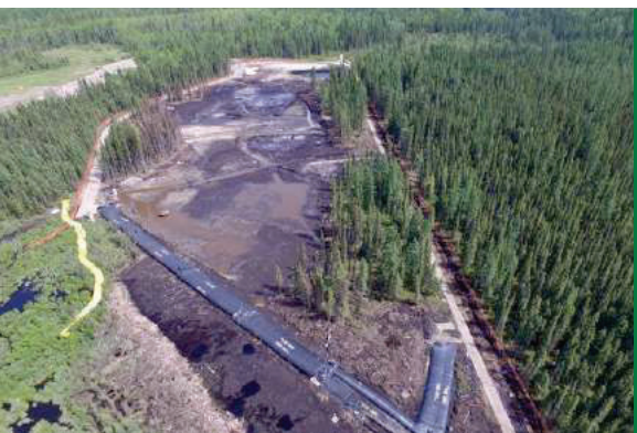
Access roads with swamp matting were constructed to access the impacted areas and point of entry from the wetland complex into the unnamed tributary. A series of terrestrial barriers were keyed into the subsoil to provide primary containment.
